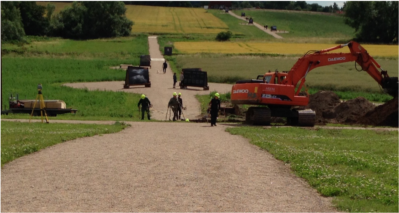
12. The water-gate of Borgring is facing South at the end of the sloping terrain where the crew, wearing yellow hard hats, are gathered. Photo: Museum Southeast Denmark.
